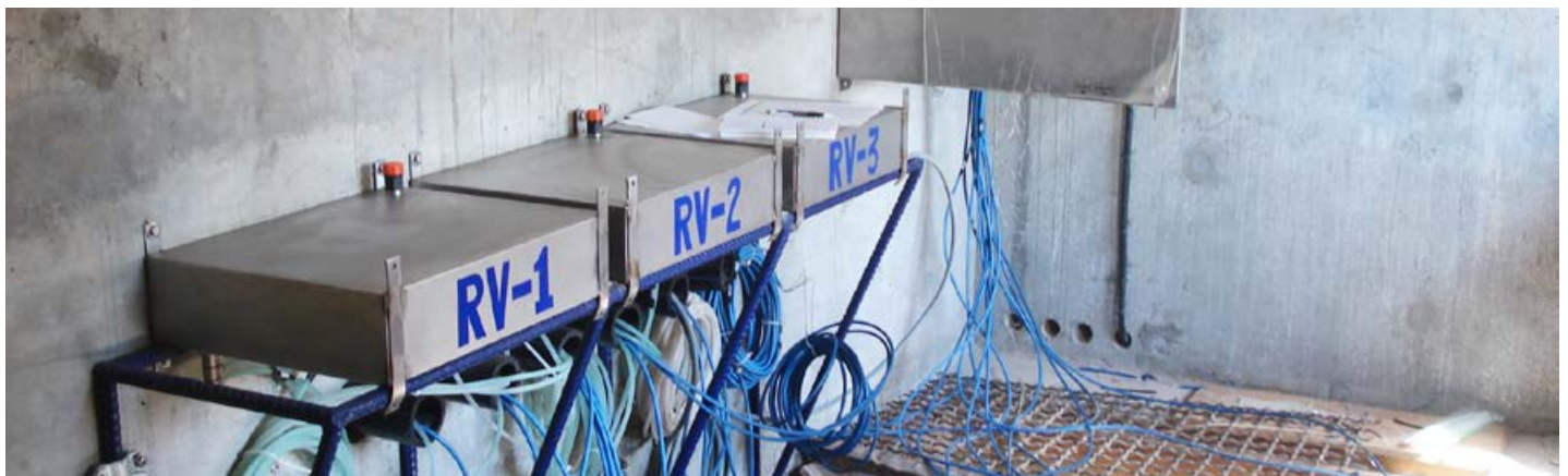
Reference vessels in Sogamoso HPP project, Colombia
