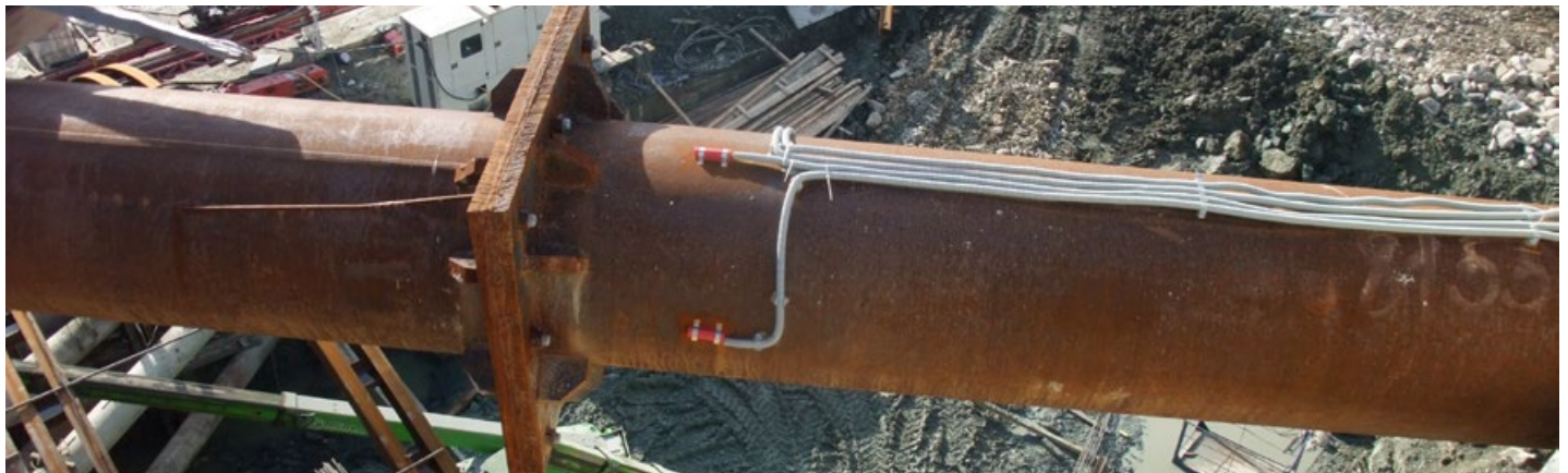
Spot weldable strain gauges on strut
